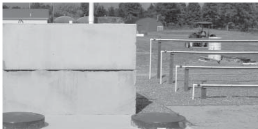
Onsite systems at the Environmental Training Center.
